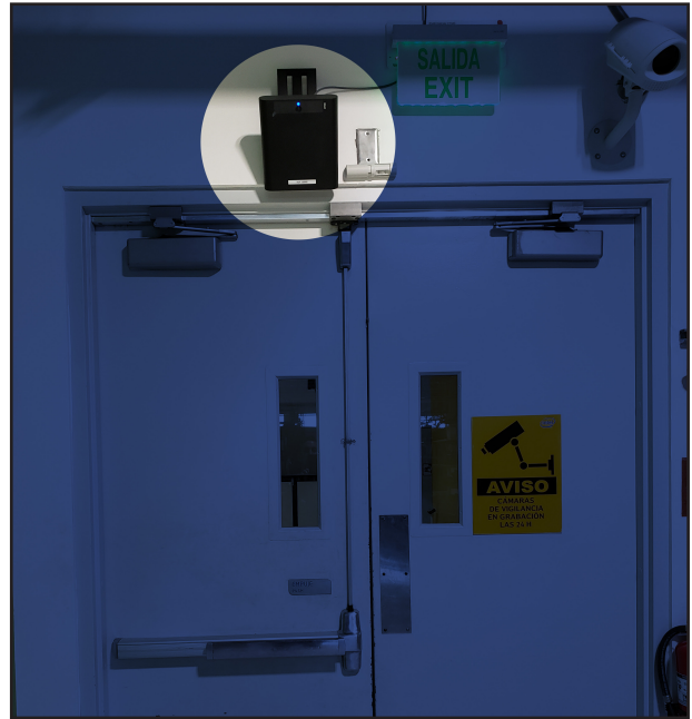
Figure 4. Sensor installed above a door
